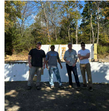
Survey Party Chief Kevin Jenkins built a new garage foundation with the assistance of several KC staff: "Thank you Benson, Mark, Chris, and Bobby for helping me. I appreciate you sacrificing your Saturdays and providing your much-needed help with this project. I also want to thank John Bolger for design assistance."
