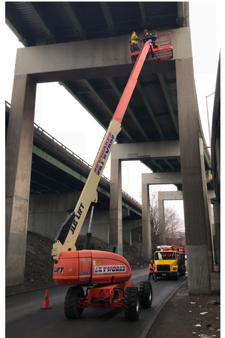
KC personnel inspecting the Bruckner Viaduct, a key interchange for I-87 and I-278.
