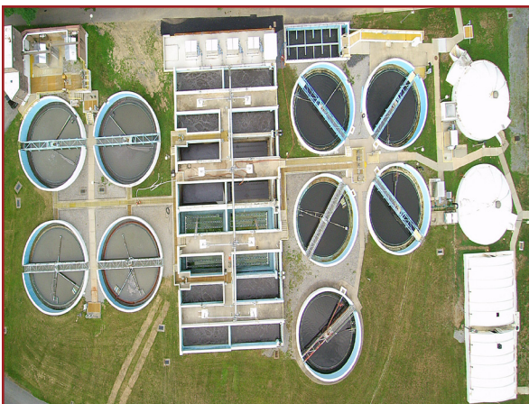
TMSC's Wastewater Treatment Plant
